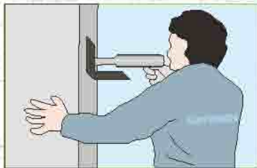
Level is obtained and bracket is fixed to column using bolt fixings
